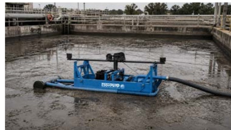
Industrial sludge basins
